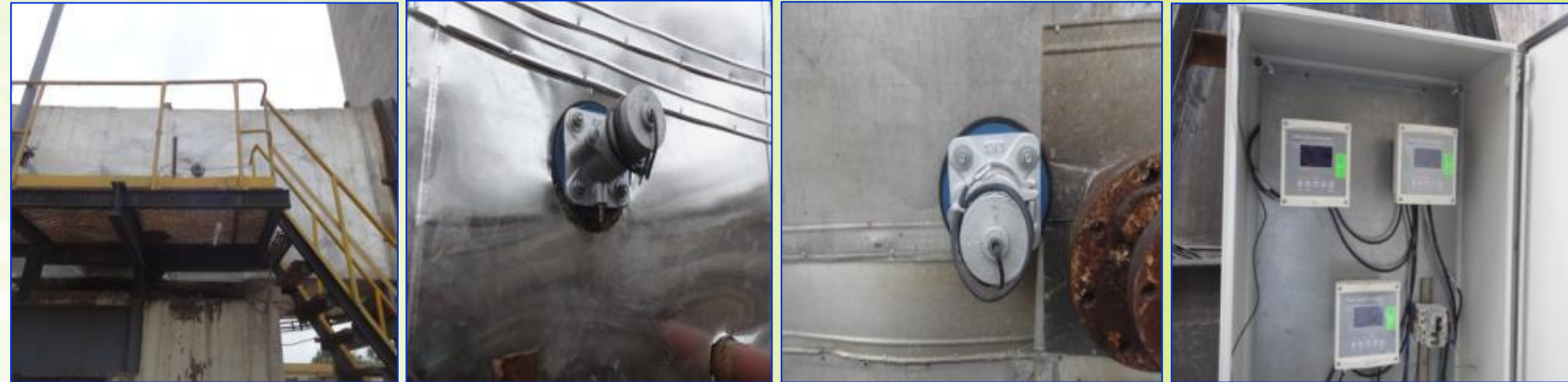
Installed Transmitter & Receiver on Boiler Duct and Local Display
