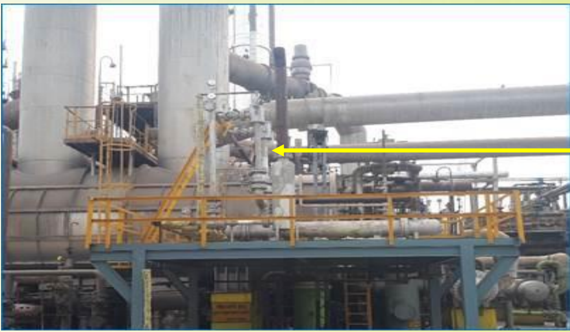
New MP Steam Ejector in Ammonia-I Plant
